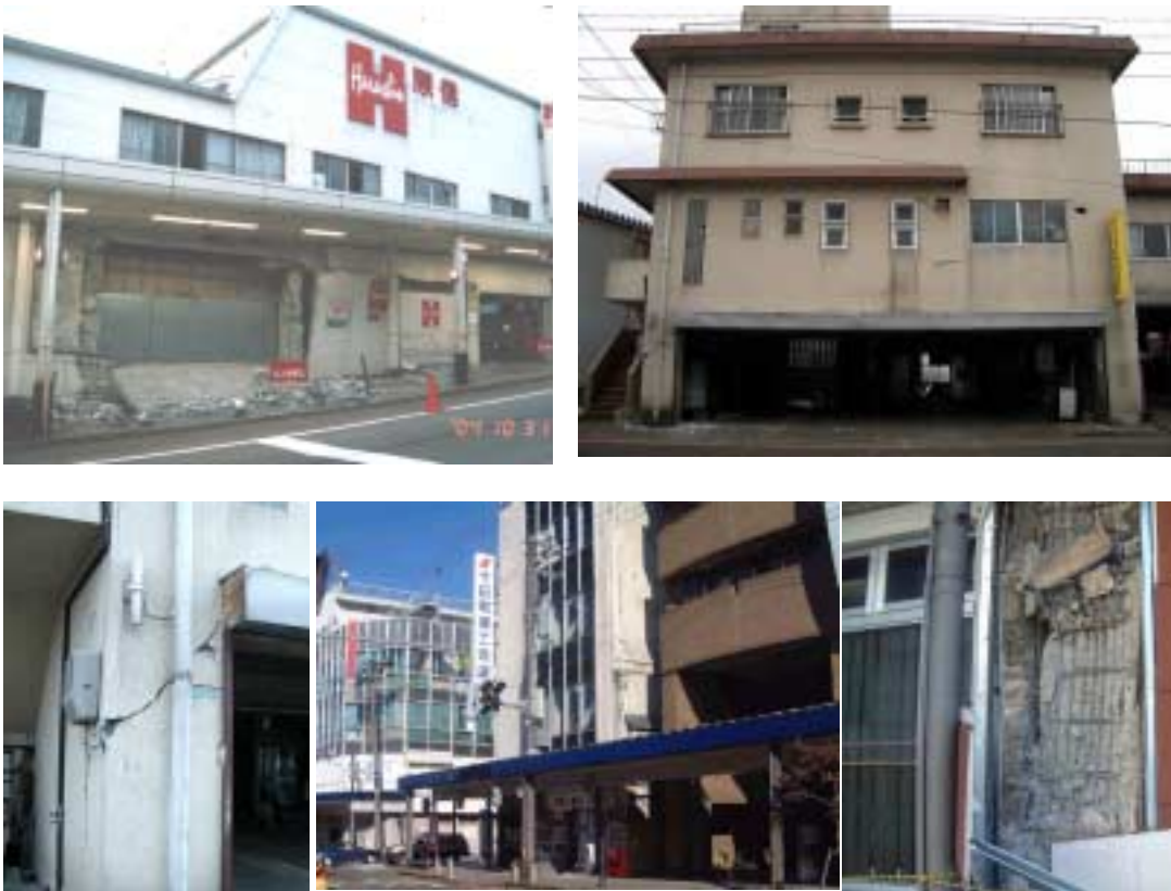
Figure 9.2: Damaged RC buildings
