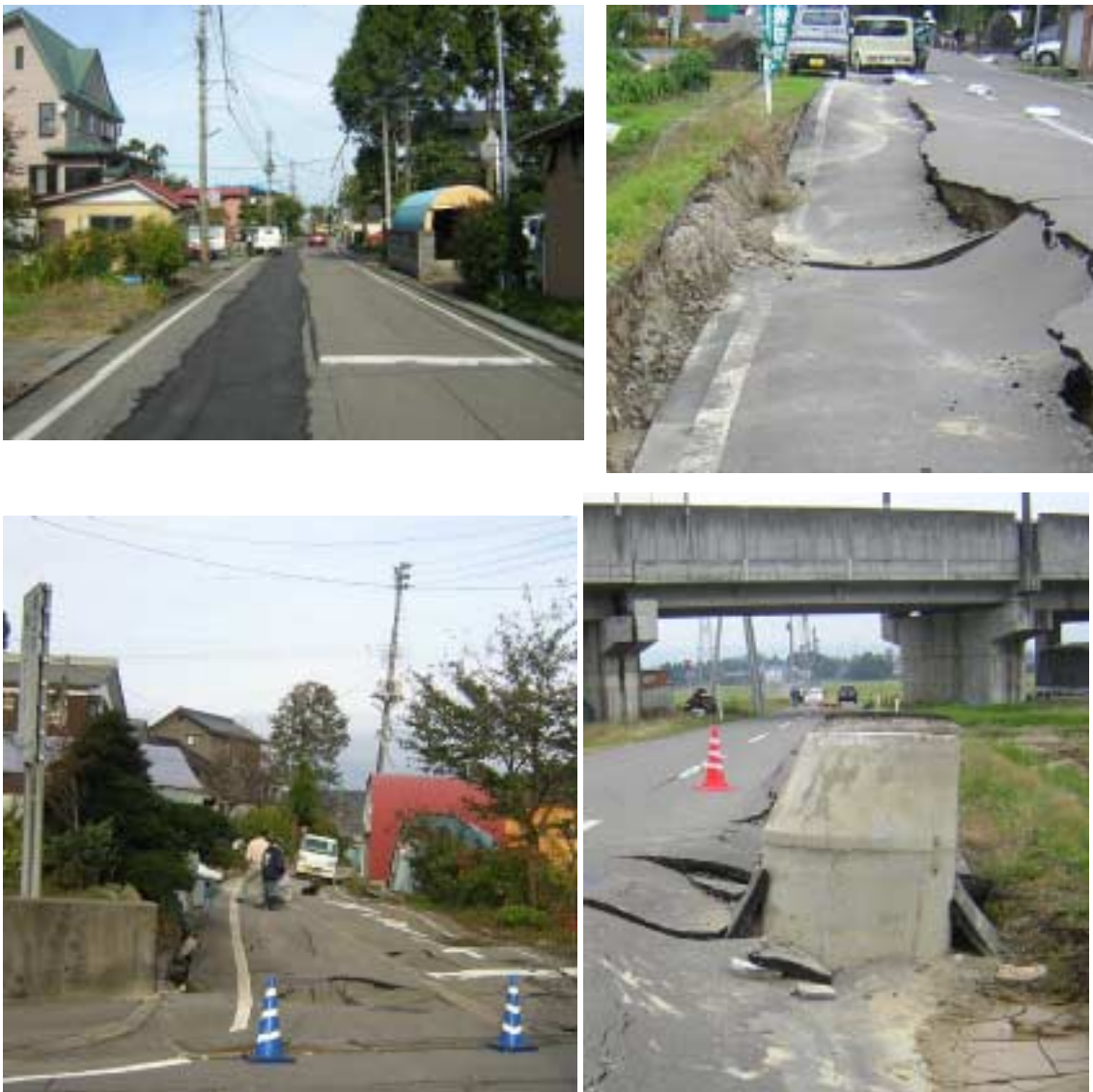
Figure 11.4: Damage to sewage systems
