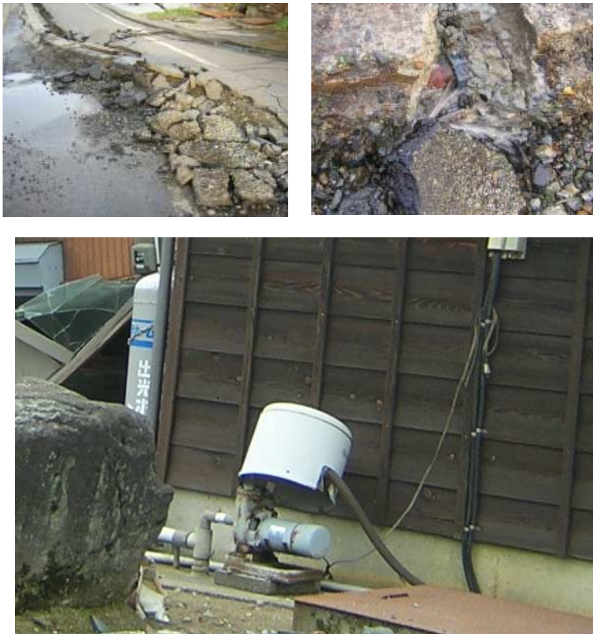
Figure 11.2: Damage to water network
